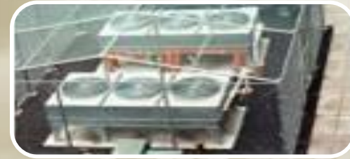
A/c – Industrial Refrigeration
